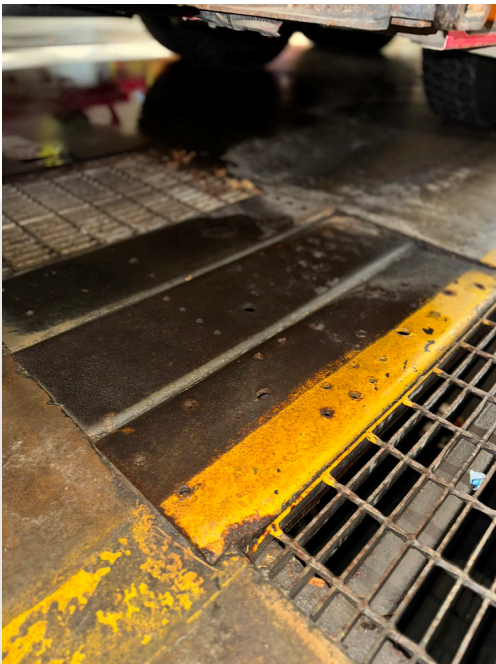
Patched in metal runners over grate at drainage pit is not structurally sound enough to hold the weight of the tanker truck- deflects significantly.
