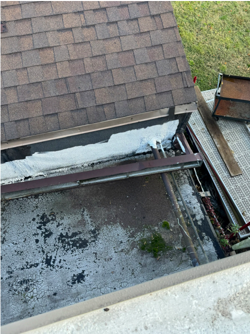
Gutter and downspout pulled away from roof edge. Plant material growing in gutters in need of repair and cleaning. Undersized downspout.
