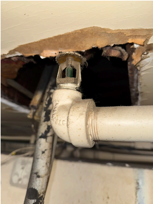
Non-functioning sprinkler system.
