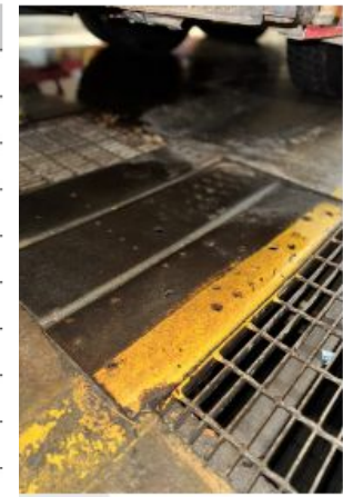
Patched in metal runners over grate at drainage pit is not structurally sound enough to hold the weight of the tanker truck- deflects significantly.
